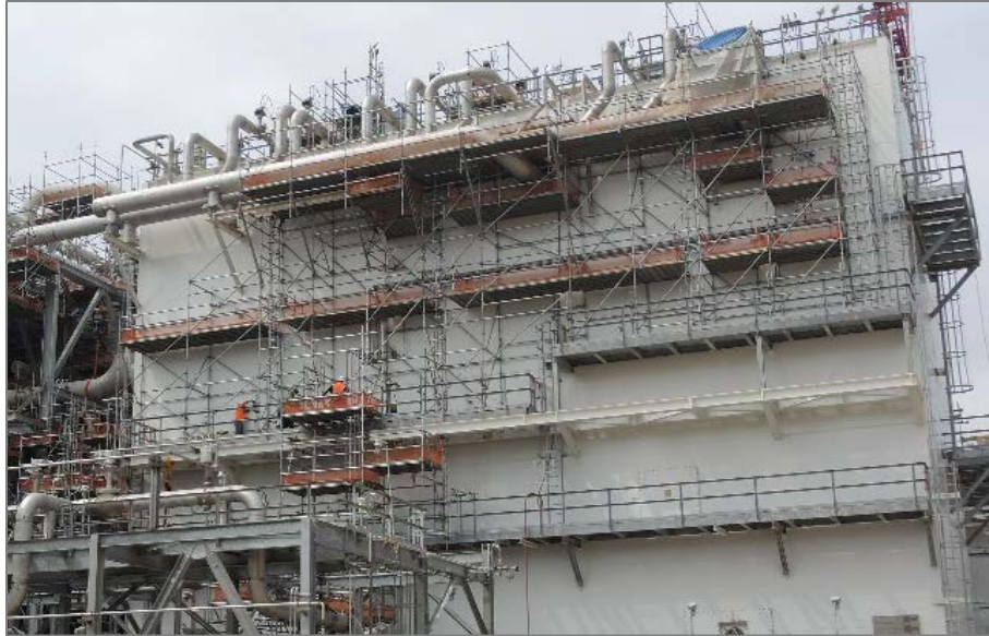
Train 4 - North Side of Methane Cold Box
