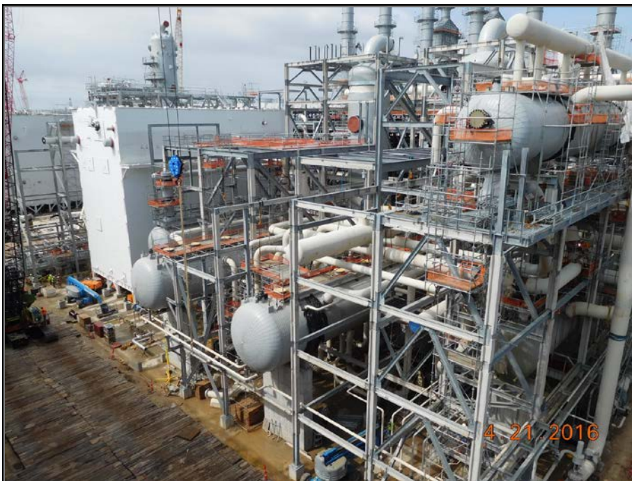
Train 4 - Propane Refrigeration Area
